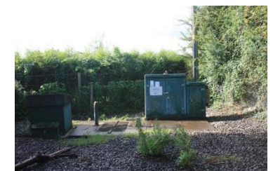
Newport pumping station
