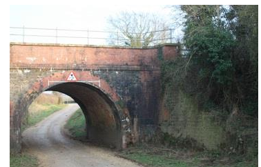
Victorian railway bridge at Damery showing the road dipping under the bridge
