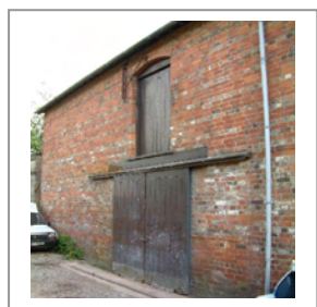
Whilst brick and stone are undoubtedly the most characteristic materials in the IHCA, the ways in which they are used and their range of textures and colours is far more subtle and complex than the ubiquitous "Stroudish" Red Brick With Stone Dressings.
