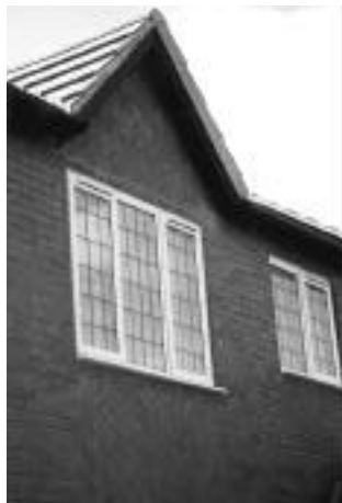
Modern windows positioned almost flush with the front of the building giving a flat, bland appearance. In addition, the cill is too thin, the proportions relate poorly to the gable and the fake leading is unconvincing and inappropriate
