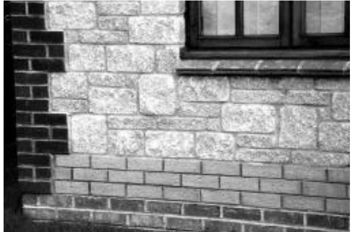
Excessive use of contrasting materials undermines local distinctiveness
