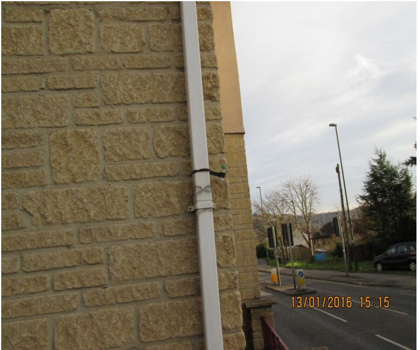
Figure 2.6 Monitoring Point 25c
